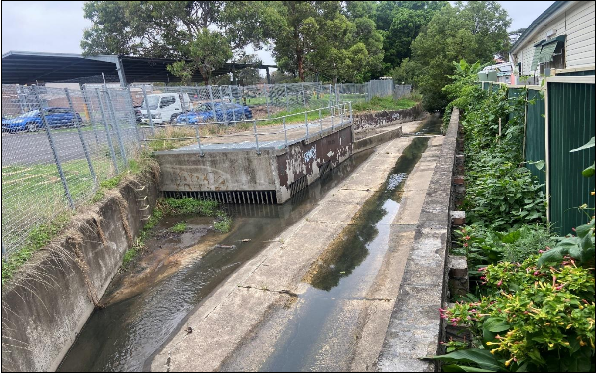
Photograph 1. Condition observed from sampling location of WP1 during the monitoring event – 22 February 2023.
