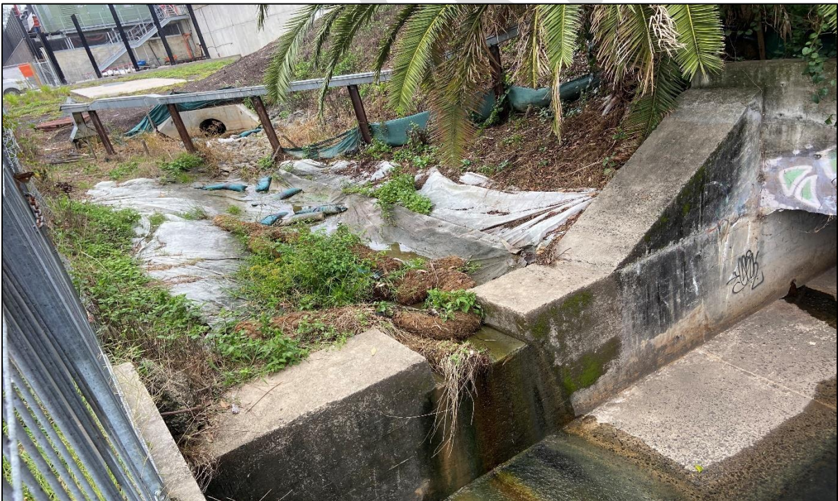
Photograph 4. High flow stormwater observed from the downstream discharge point WP2-DP1 which were located within the rail corridor and immediately upstream / south from WP2 during the monitoring event – 22 February 2023.
