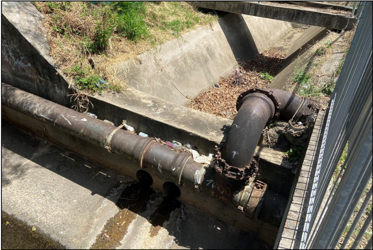
Photograph 5. No stormwater in-flow observed from the downstream discharge point WP2-DP2 which were located within the rail corridor and immediately upstream / south from WP2 during the monitoring event – 25 November 2022.
