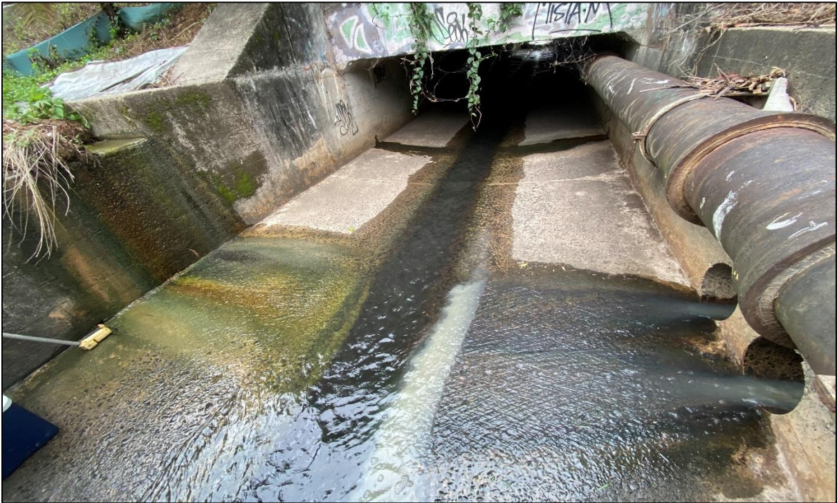
Photograph 5. High flow stormwater observed from the downstream discharge point WP2-DP1 which were located within the rail corridor and immediately upstream / south from WP2 during the monitoring event – 22 February 2023.
